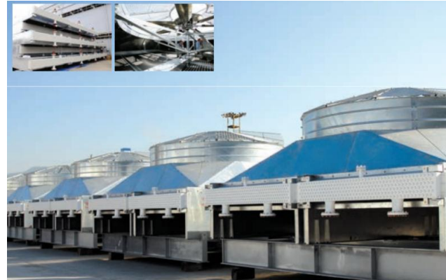
Air Cooled Heat Exchanger
